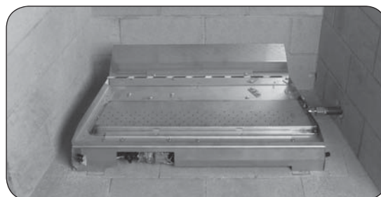
Fig. 14-2 Center burner in fireplace
